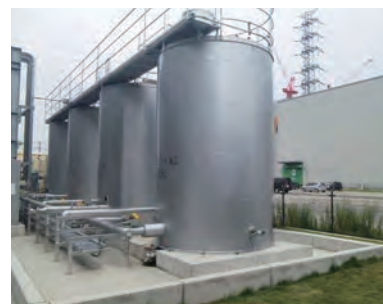
Liquid storage facility
