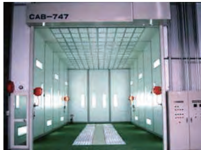
Large airframe painting/drying booth
