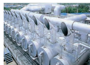
Solvent recovery equipment
