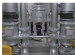
Noxious gas abatement equipment
