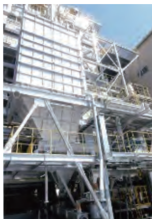
Sand circulation equipment
