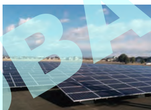
Solar power system
