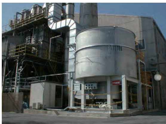
4 Deodorization Equipment (Kondoh Industries)
