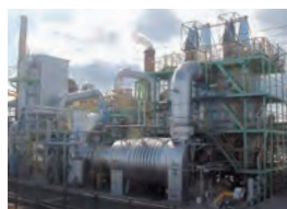
Dry distillation gasification incinerator
