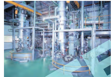
Liquid polymerization plant
