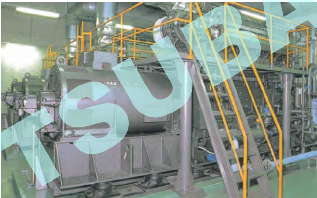
③ Cogeneration Equipment (Tess Engineering)
