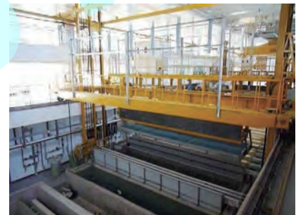
Automatic surface processing equipment, fluorescent penetrant inspection equipment
