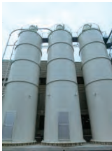
Silo for bulk materials Stores raw material unloaded from a bulk truck.
